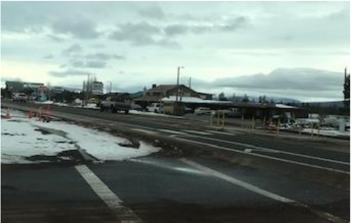
Figure 13. US 97/Finley Butte Road intersection facing south showing the newly installed raised pedestrian refuge island and sidewalks.
